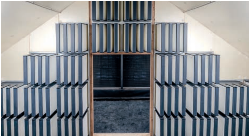
Flexible filter frame system and pad cooling
