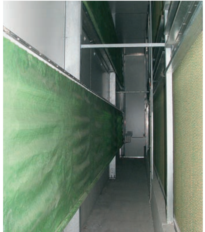
Tunnel inlet with roller curtain
