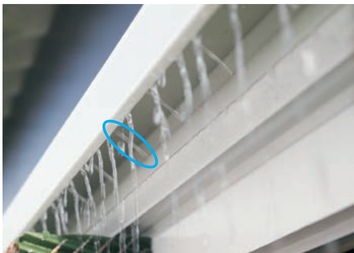
Top profile with perforated pipe and deflector for an even distribution of water along the pads
