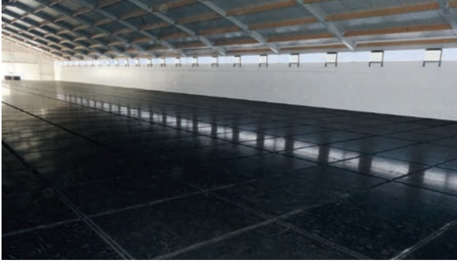
View of an intermediate ceiling made of plastic panels before the system is installed on the second level
