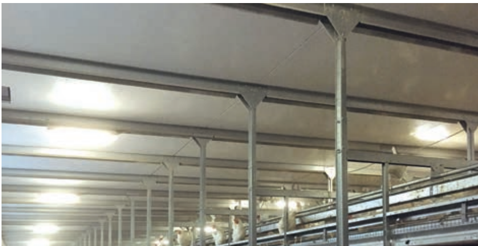
The smooth, white surface of the plastic panels' underside allows fresh air to flow crosswise through the house without obstructions
