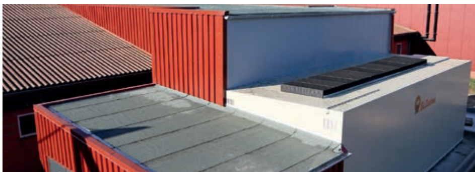
Retrofitted Porcus air scrubber
